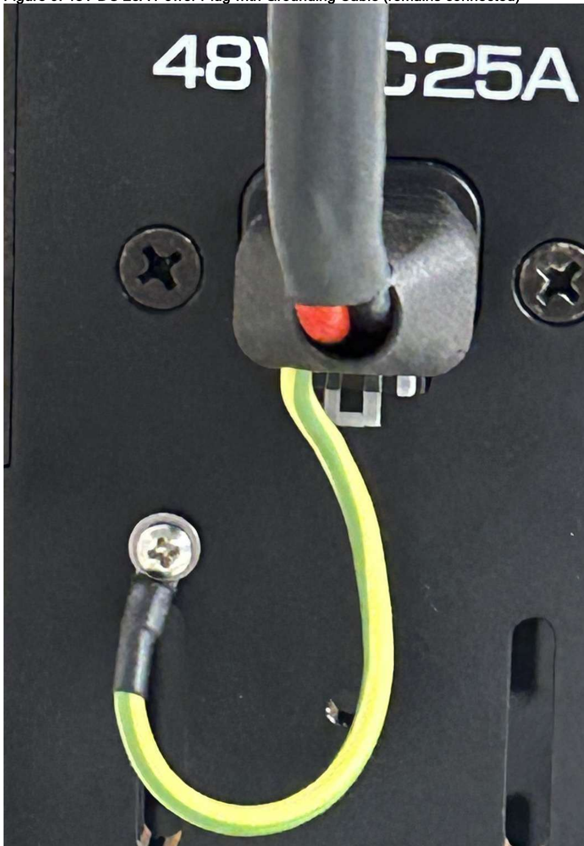
Figure 9: 48V DC 25A Power Plug with Grounding Cable (remains connected)
