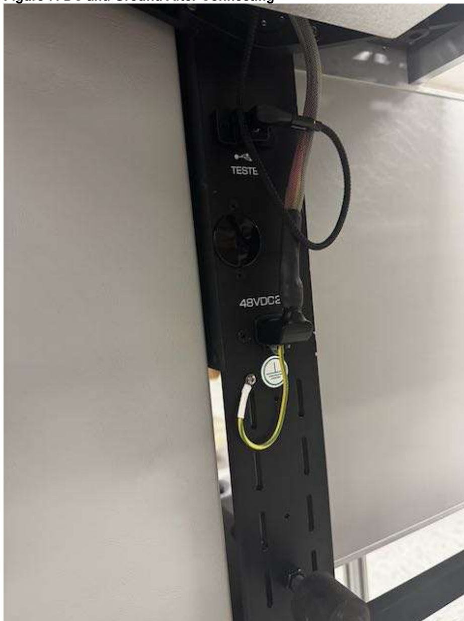
Figure 7: DC and Ground After Connecting
