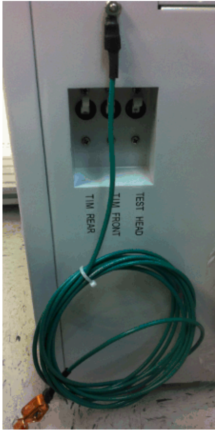
Handler Grounding Wire
